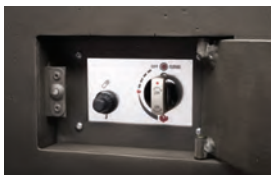
Concealed Control Panel
