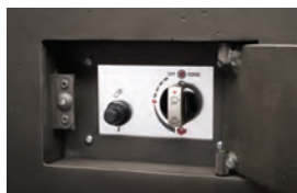
Concealed Control Panel
