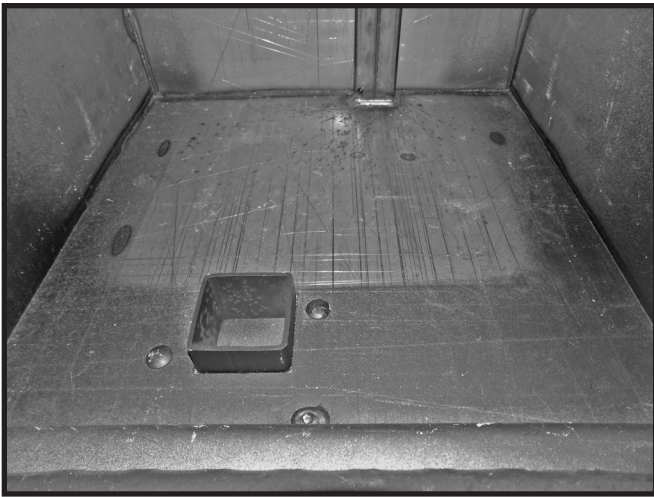
Figure 14: Floor of firebox and ash dump.
