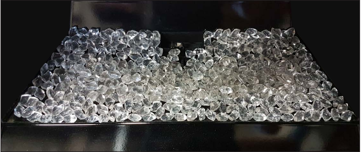
Figure 55: Burner tray with glass media installed.
