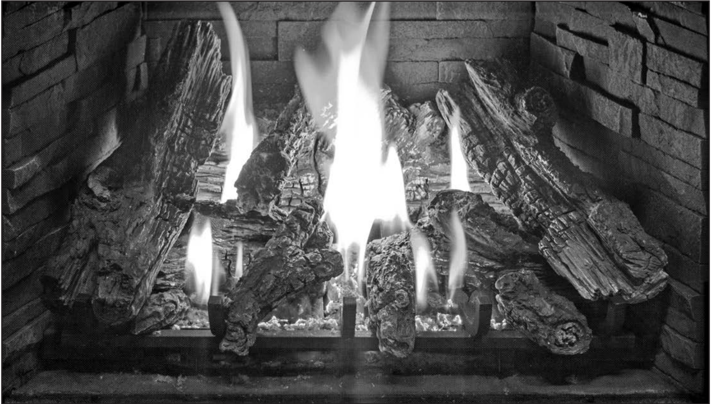
Figure 63: Proper installation and flame appearance
