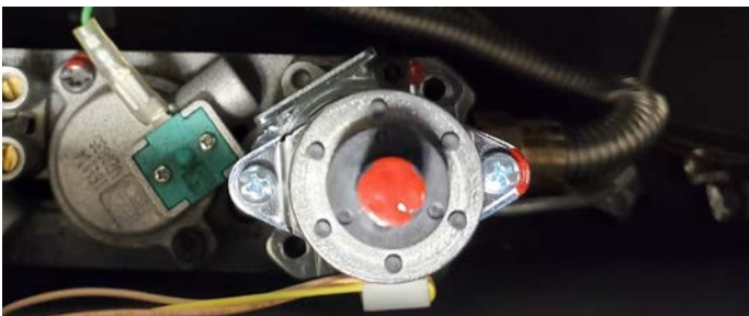
Figure 13.eee LP pressure regulator on a Full Load
