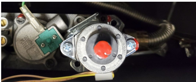
Figure 13.eee LP pressure regulator on a Full Load
