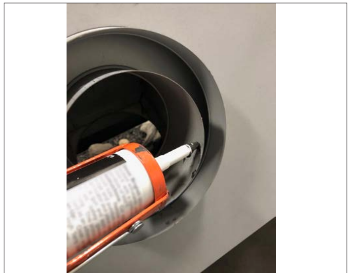
Figure 2.2, Silicone Inner Exhaust on Fireplace
