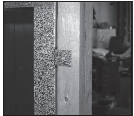
Figure 20: Framing tabs bent out.
