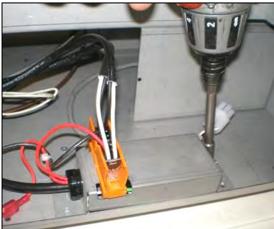
Lamp Transformer housing may need to be moved toward valve.
