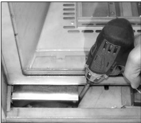
Power Vent Control Module Mounted inside fireplace.
