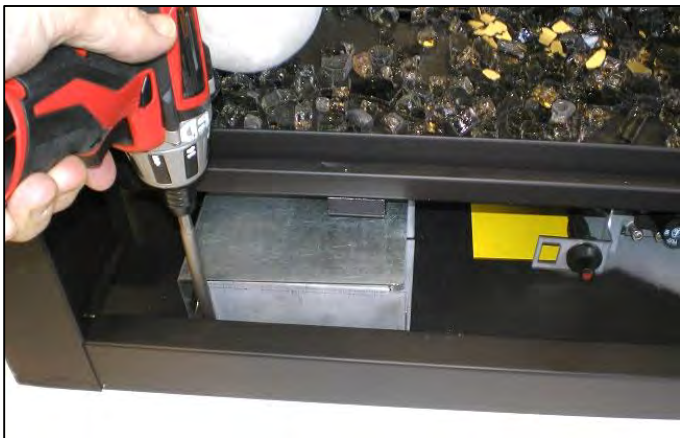
Power Vent Control Module Mounted inside fireplace.
