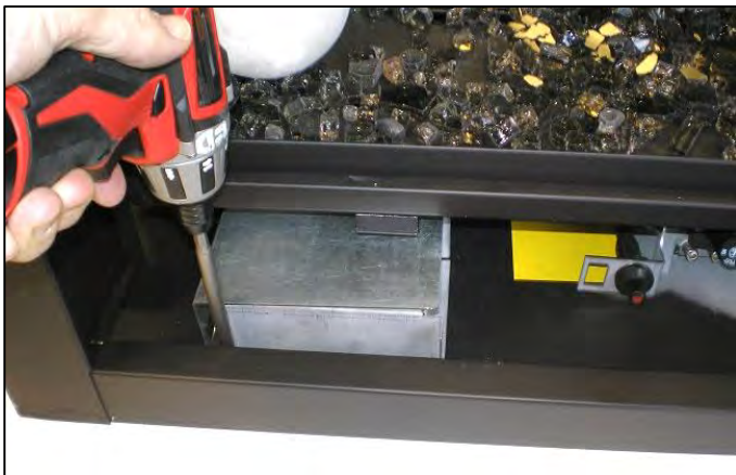
Power Vent Control Module Mounted inside fireplace.
