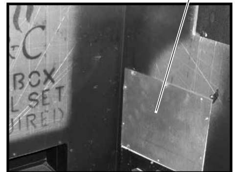
Figure 22: Access to firebox.
