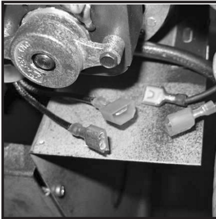
Figure 13: Disconnecting fan wires.
