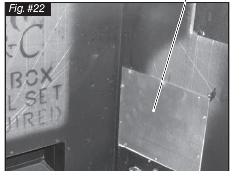
FIREBOX ACCESS PANEL
