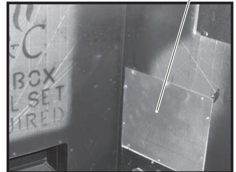
Figure 22: Access to firebox.
