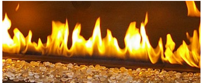
Figure 25a. Operating gas fireplace with firestones surrounding burner tray.
