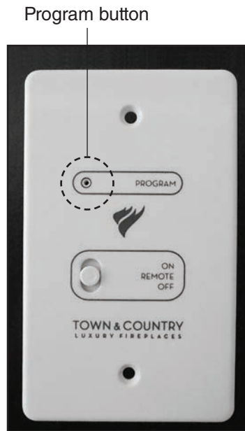
Figure 59: T&C Wall switch plate.
